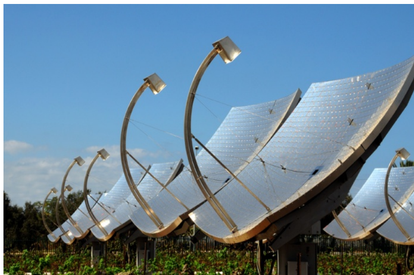
ZenithSolar Z20 CHP Solar Technology installation successfully operating at KibbutzYavne Israel since April 2009
