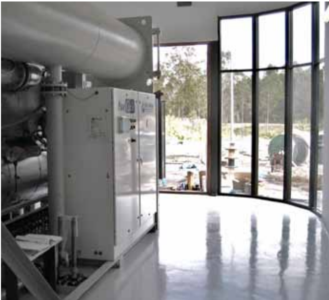
Figure 5: 280kW Purecycle ORC power system installed at Gympie Timber to convert sawmill residue into electricity
